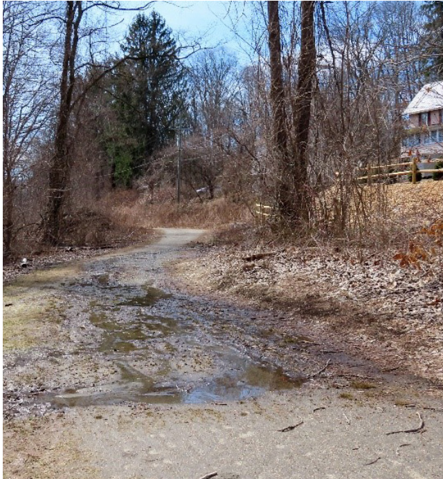
ALSPT Trail surface erosion from rain event
