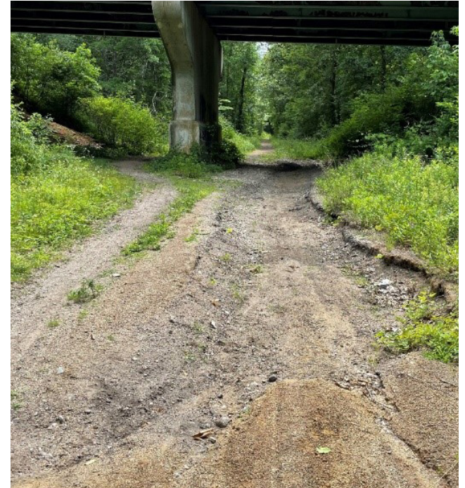
Trail erosion from highway stormwater in Thompson
